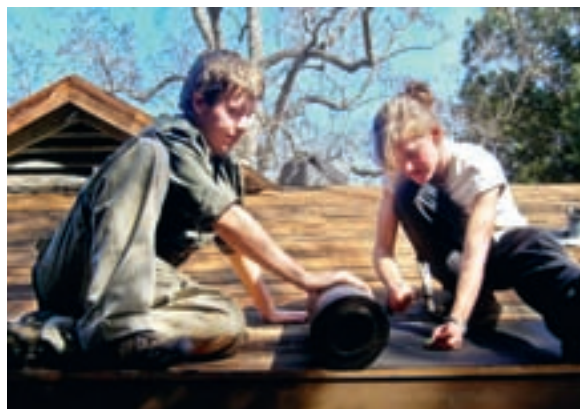
Jotham Penner of Kitchener and Noelle Koop of Winnipeg work on a roof in Mobile, Alabama.
